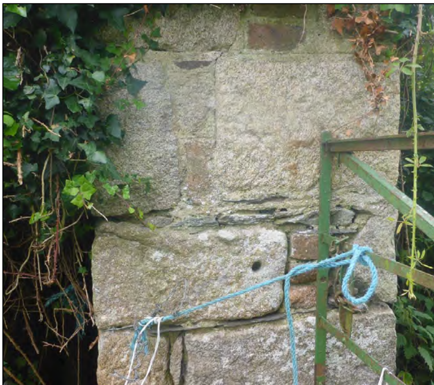
Plate 6 Detail of southern gate pier, showing drilled hole for original gate fixings
